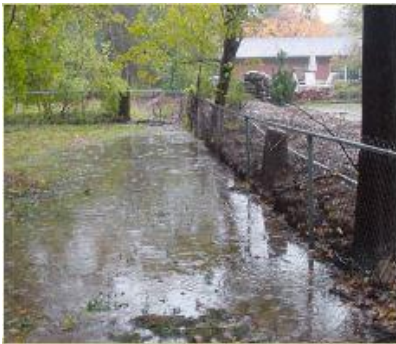
Blocked Drainage Swale
